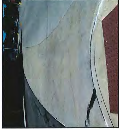
Missing sidewalk at Westwood Drive
